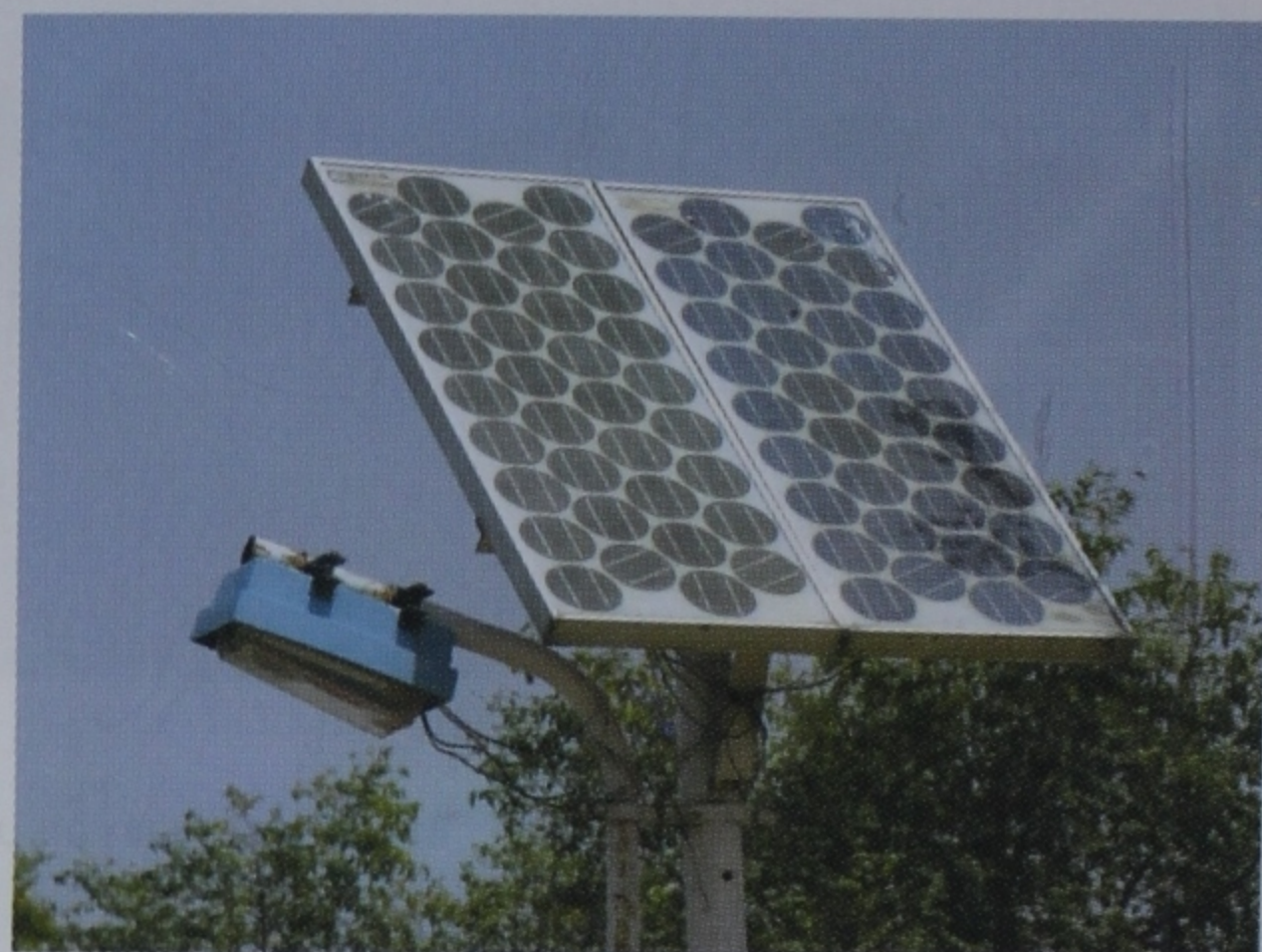
Fig. 4.13 Solar panels are used for lighting.
