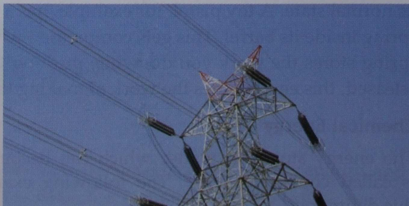
Fig. 4.9 Electricity can be transported easily.
